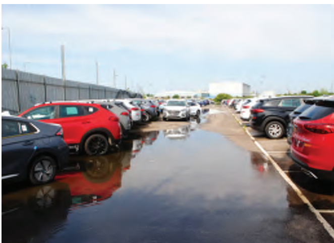
Location 9: Looking W across Compound C. Poor drainage evident
