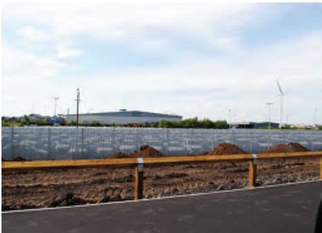
Location 6: Looking S across car storage at C Compound. Unit 1 in background
