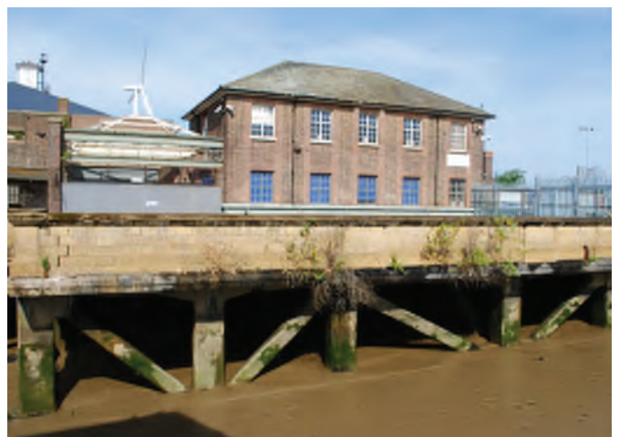
Location 3: Looking W at Cultural Centre (E end of Rail Station building)
